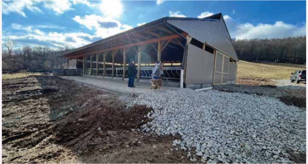
The photo above shows a roofed heavy-use area that was installed, the picture does not show the completed project.
