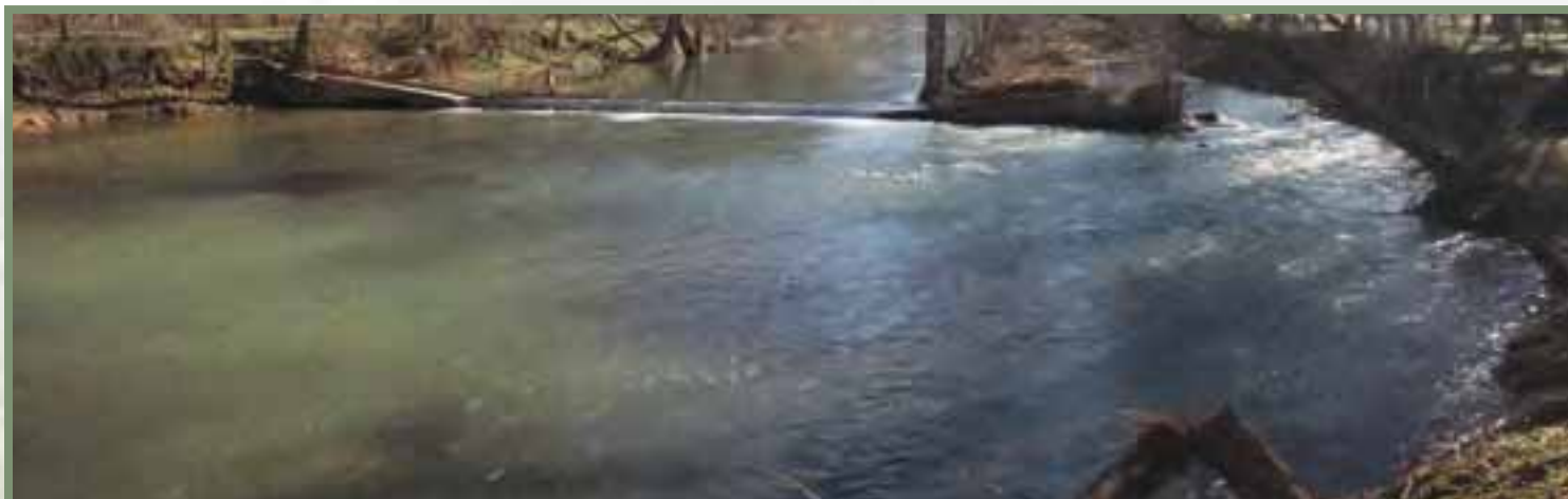
This pre-construction photo, taken from the northern streambank, shows the collapsed bridge disconnected from the opposite bank. A secondary stream channel had formed to the right, diverting water during high-flow events. When water levels rose, the stream spilled over the remains of the structure, increasing safety risks and contributing to ongoing erosion.
